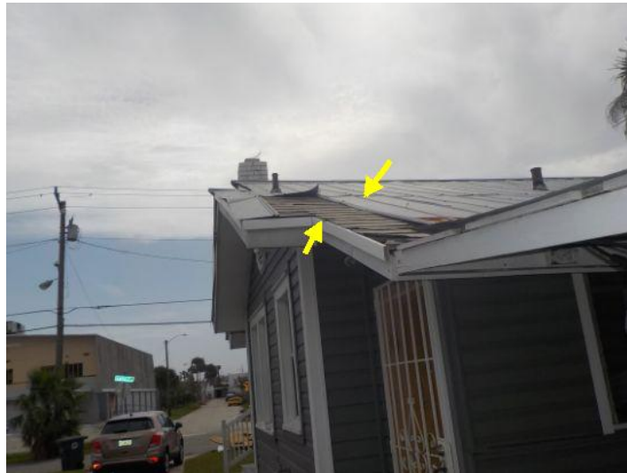
Roof Roof damages
