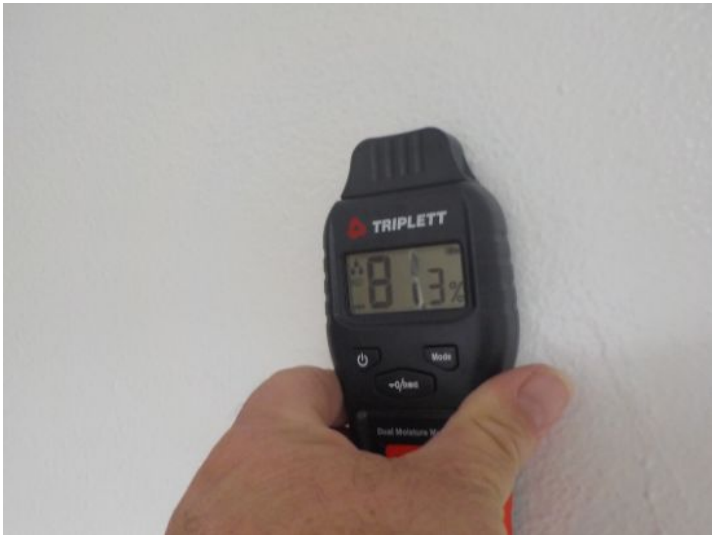
Advise remove and discard 2" of drywall from floor up until clean margins have been achieved.
