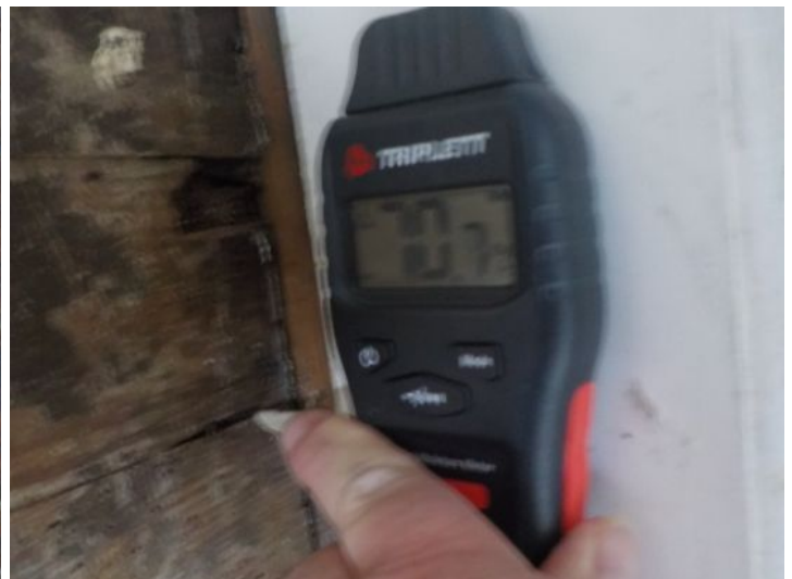
Advise remove and discard 2" of drywall from floor up until clean margins have been achieved.
