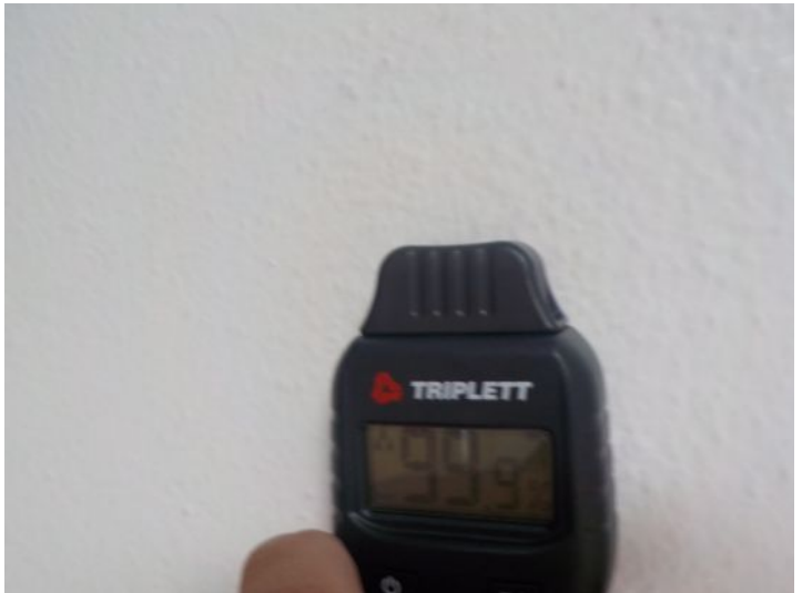
Advise remove and discard 2" of drywall from floor up until clean margins have been achieved.
