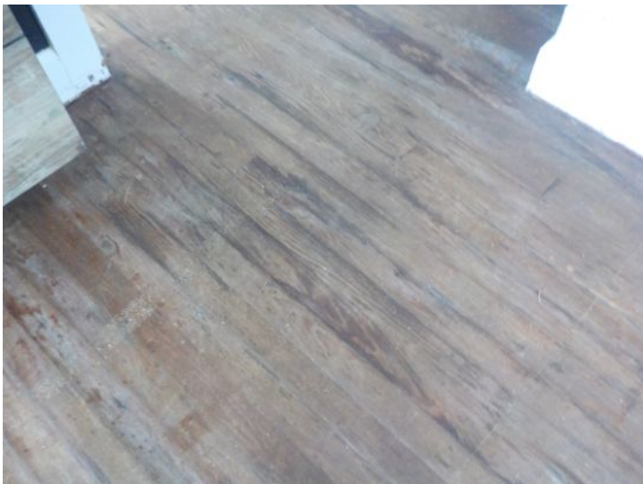
Advise removal of 100% wet floor covering in the living room area.
