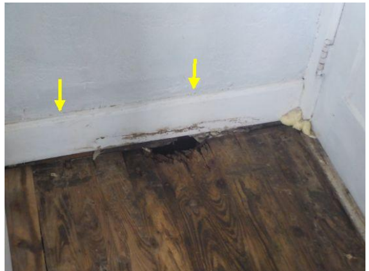
Advise remove/and discard all base moldings in living room area.
